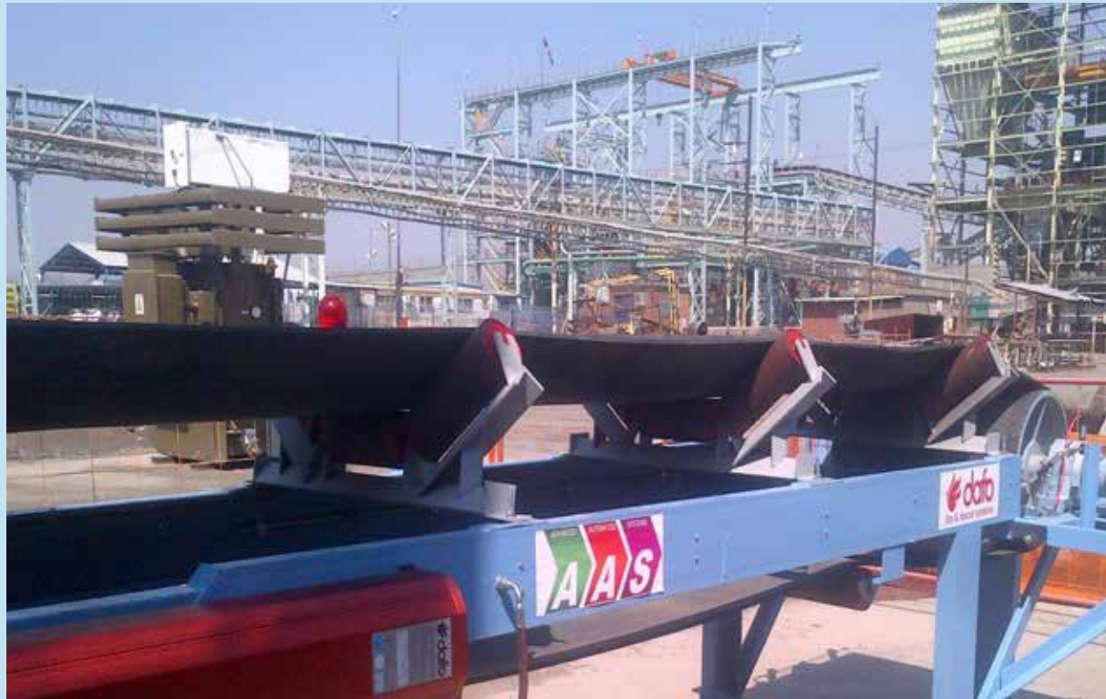
Mock-Up Conveyor with Delta Detector and Forrex System Installed
